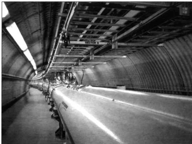
RHIC magnets, a view inside the RHIC ring tunnel. Photos courtesy of Brookhaven National Laboratory.
